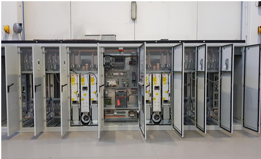
Figure 1 – Drives fitted in the control panel for the project.
