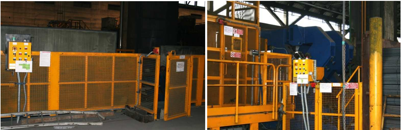
Fig. 10. Left: Safety gate with electric lock open; green light over the local box means safety access. Right: gate closed (the machines of this area are running); red light means forbidden access.
