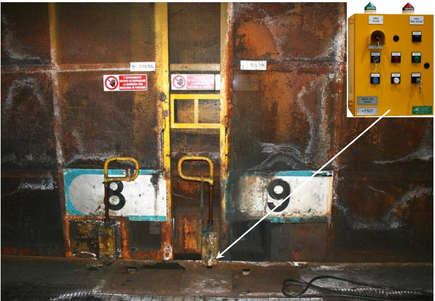
Fig. 11. Sliding shields (ahead finishing stands) controlled through electric bolt unlocked from safety control accesses.
