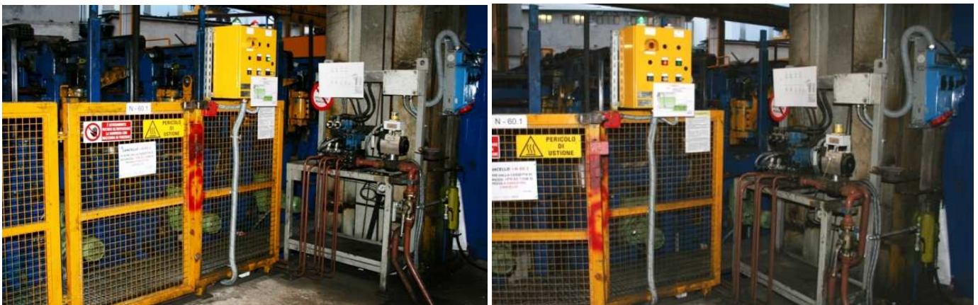
Fig. 17. Safety system applied on hydraulic devices and distribution: hydraulic bank, main delivery block valves controlled by local safety box and pressure decay control.
