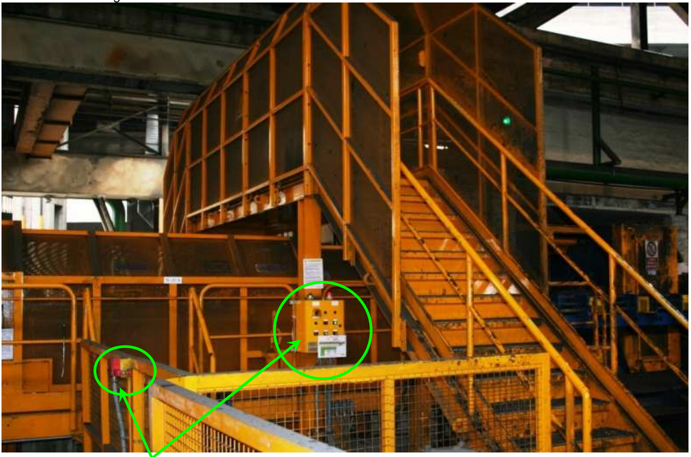
Fig. 9. Close-up: Safe gate with electric lock controlled by safety dedicated local box. Behind: fixed (passage protections) and sliding security shields (in front of rolling machines)
