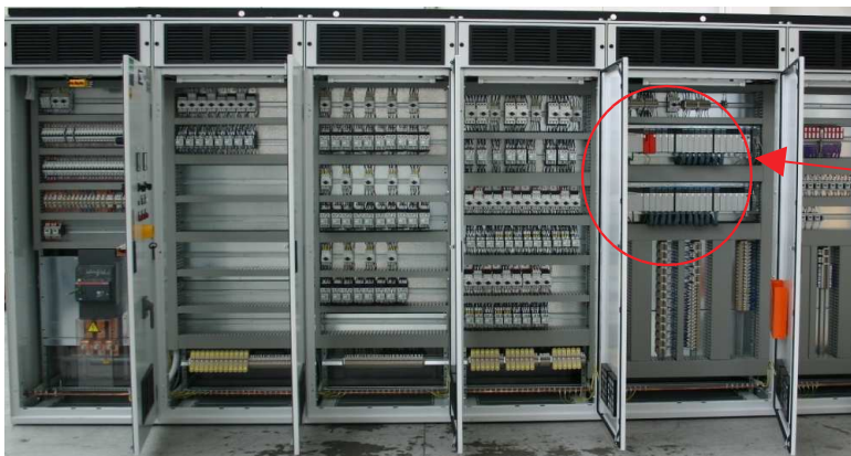
Fig. 8. Auxiliary Services Panel with Safety CPU
