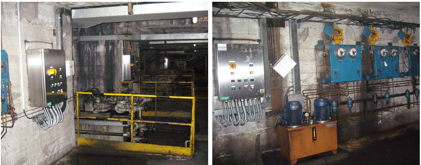
Fig. 17. New local stations suited to control oil circuit
