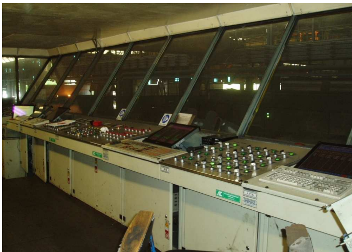
Fig. 9. Main control room (Rolling mill area) before revamping
