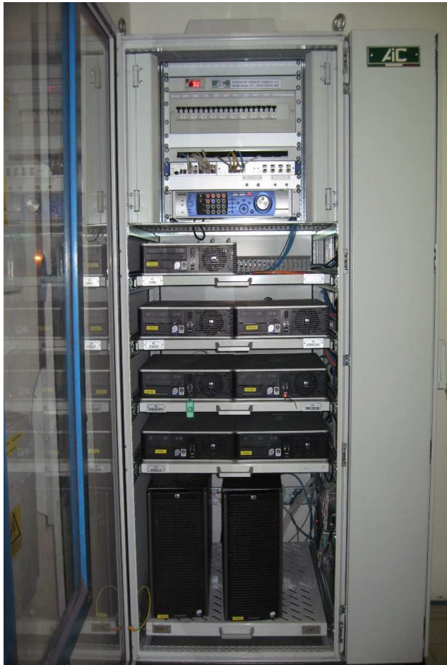
Figure 22: PC Panel with client/server IT machines and CCVE digital recorder
