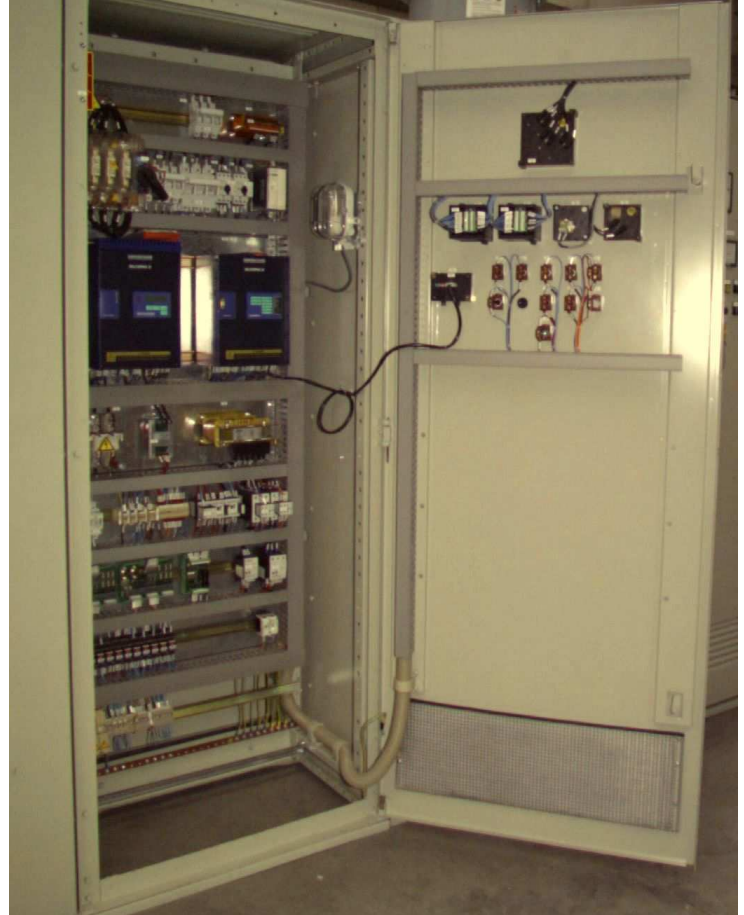
Fig. 7. Sample of DC Drives after revamping
