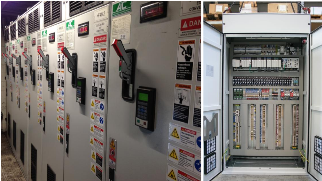
Fig. 5-6: New VFD drives and ControlLogix PLC supplied by AIC
