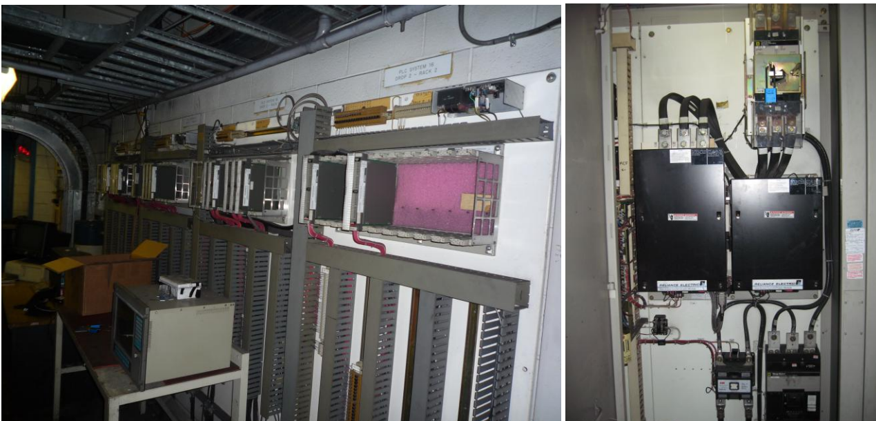
Fig. 3-4: Existing Modicon PLC and DC Drives before AIC revamping
