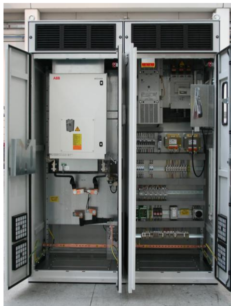
Fig. 7: One of the new DC Drives supplied by AIC
