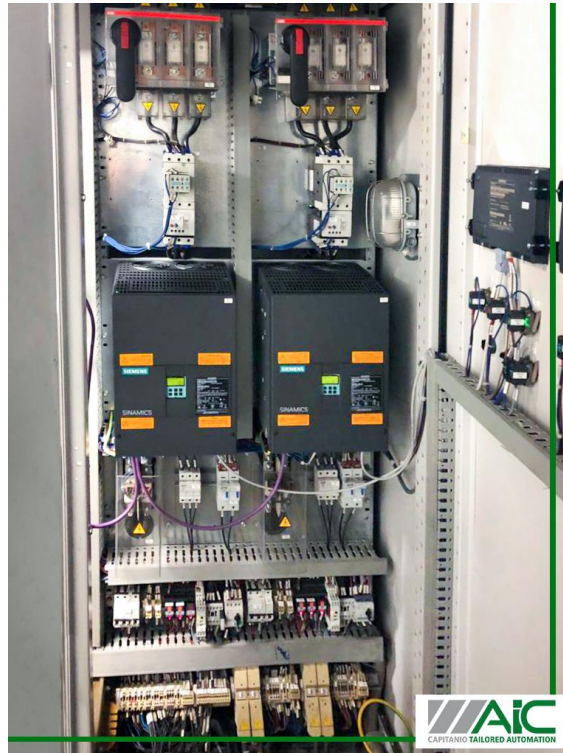
2 Siemens Sinamics DCM 210A converters installed in the cabinet
