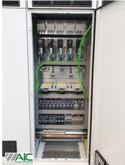
Fig. 2 The extension of the control panel
