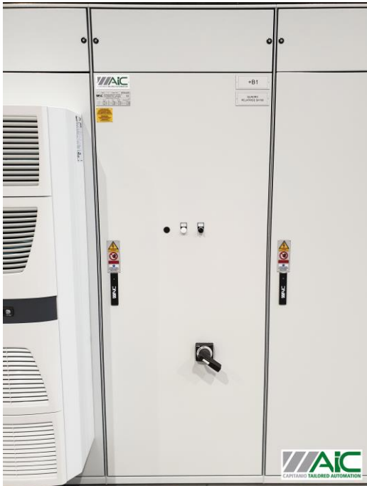
Fig. 1 Control panel installed at the beginning of 2020
