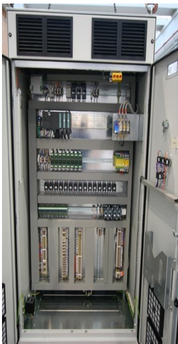
PLC Cabinets supplied by AIC
