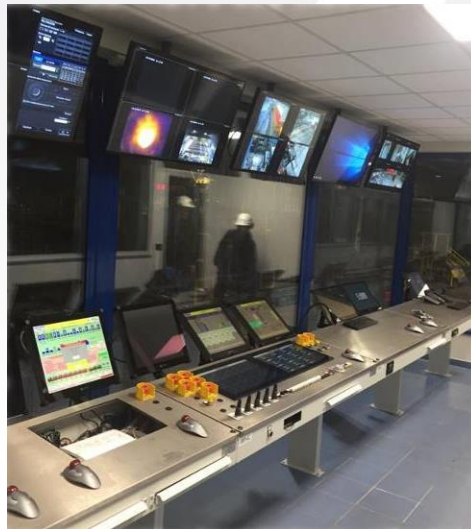
The example of the main pulpit for the control of the rolling mill
