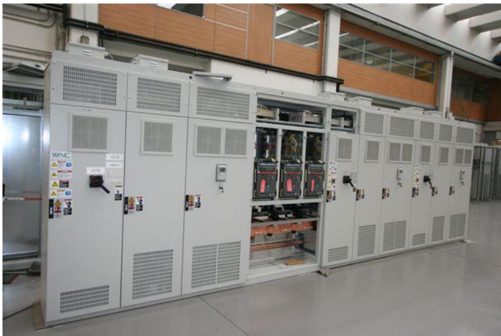
Drive panels supplied by AIC to Cascade Steel
